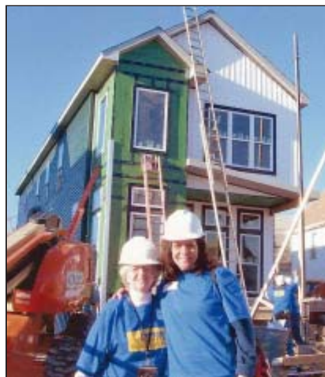
Wearing hardhats, Pauline and niece, Carolyn Baach, stand in front of the house being "made over." They were among 5,000 volunteers.
