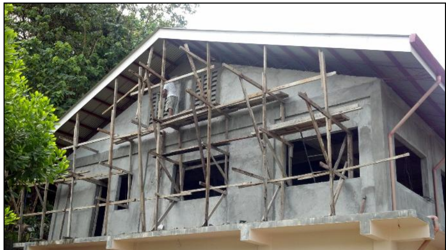
In the photo is a side view of the Speech Lab side view facing Holy Cross Convent. The facility, still under construction, replaces the one destroyed in the fire.
