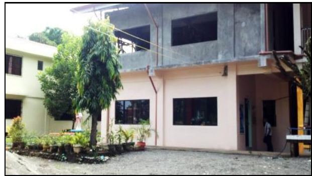
Here is a photo of the newly finished Faculty Room to replace the burned one. The second story, which will house the Speech Laboratory destroyed in the fire, remains under construction.
